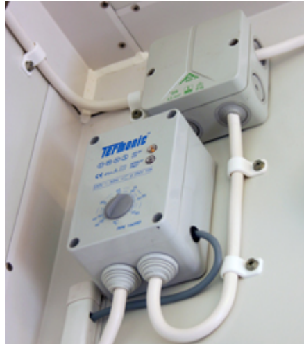
Figure 9: Thermostatic and Junction box
