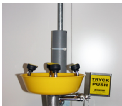
Figure 6: Plastic pipe to drainage
