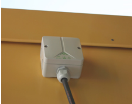
Figure 8: Assigned place for electricity
